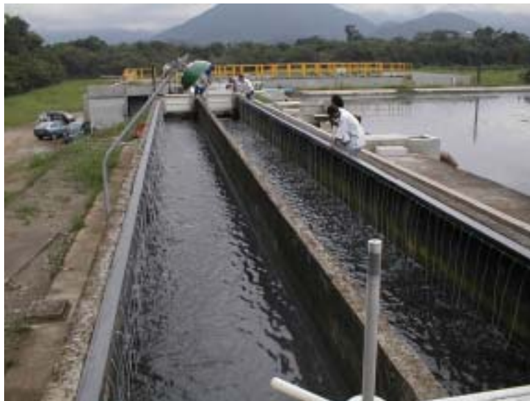
Figure 9: Flocculation Chambers (23m long)
