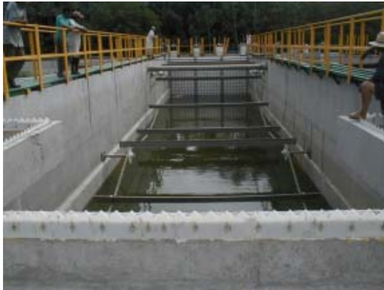
Figure 11: CEPT Tank and the Sludge Scrapers
