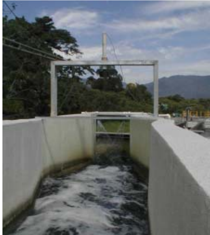
Figure 19: Parshall Flume, Ultrasonic Sensor, and Polymer Dosing
