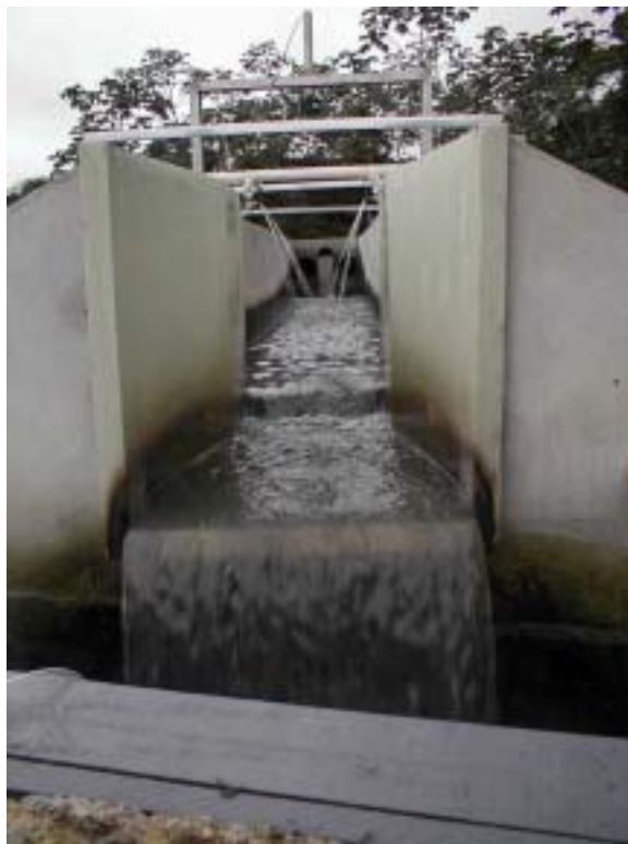
Figure 22: Sampling Point I-2, Influent Parshall Flume
