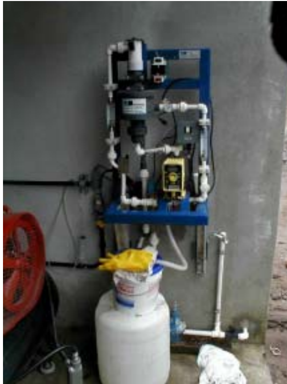
Figure 20: Polymer Pump and Dosing System
