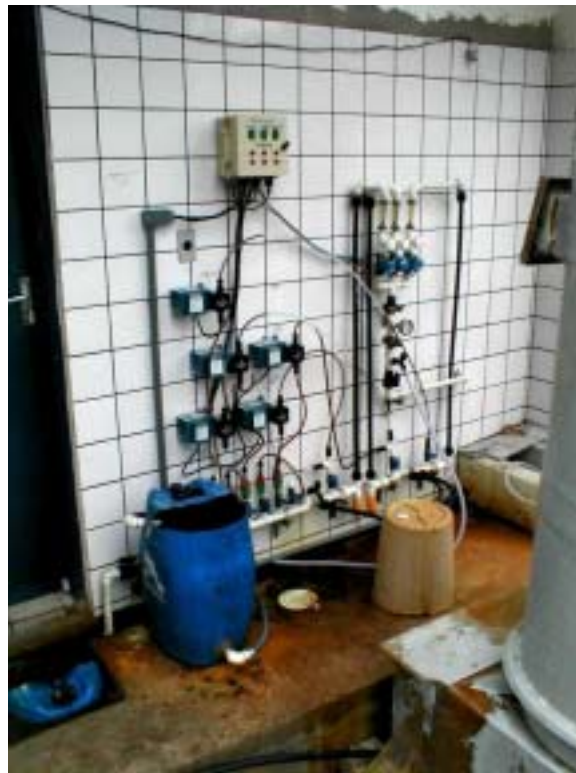
Figure 17: Metal Salt Dosing System
