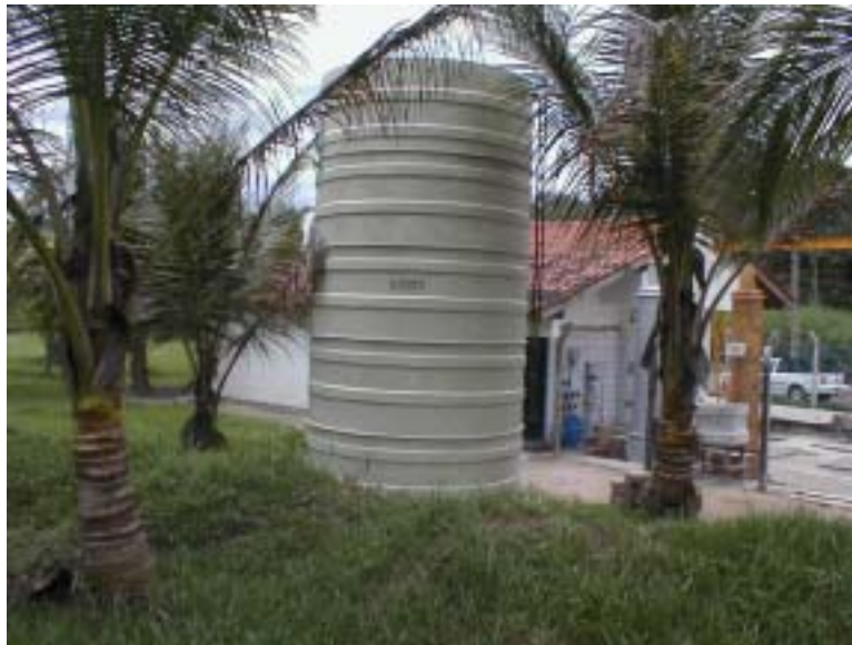
Figure 16: Chemical Storage Tank
