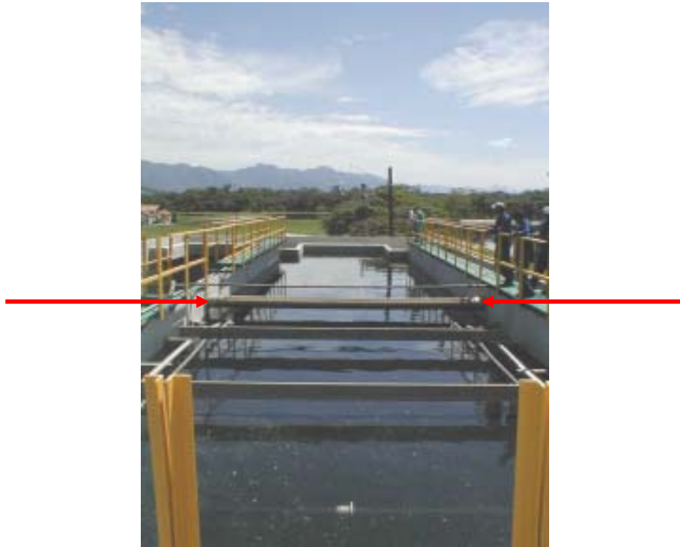
Figure 12: Scum Scraper Located at the Surface of the Clarifier Tank
