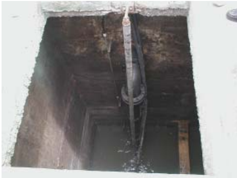
Figure 18: Metal Salt Injection into the Pump Well
