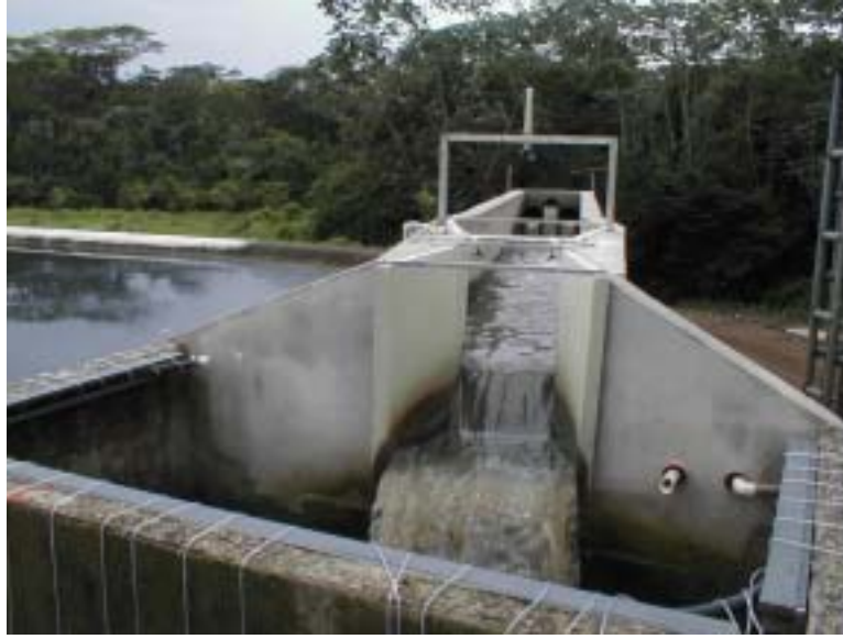
Figure 7: Feed Channel, Parshall Flume, Flow Meter, and Polymer Dosing
