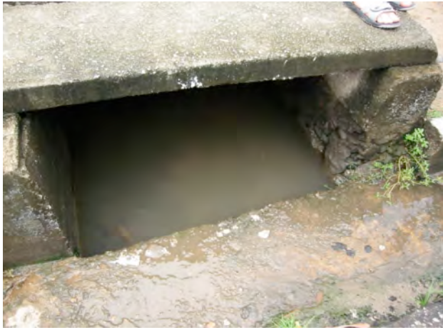
Figure 1.9: Dilute sewage in an open ditch
