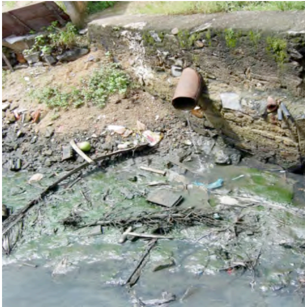
Figure 1.7: Sewage Discharge into Street (2)
