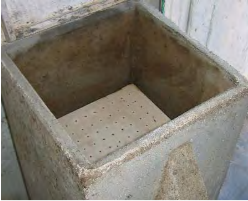
Figure 3.4: A diffuser plate inside a BioSand Filter in the Dominican Republic. Source: Heather Lukacs, 2004.
