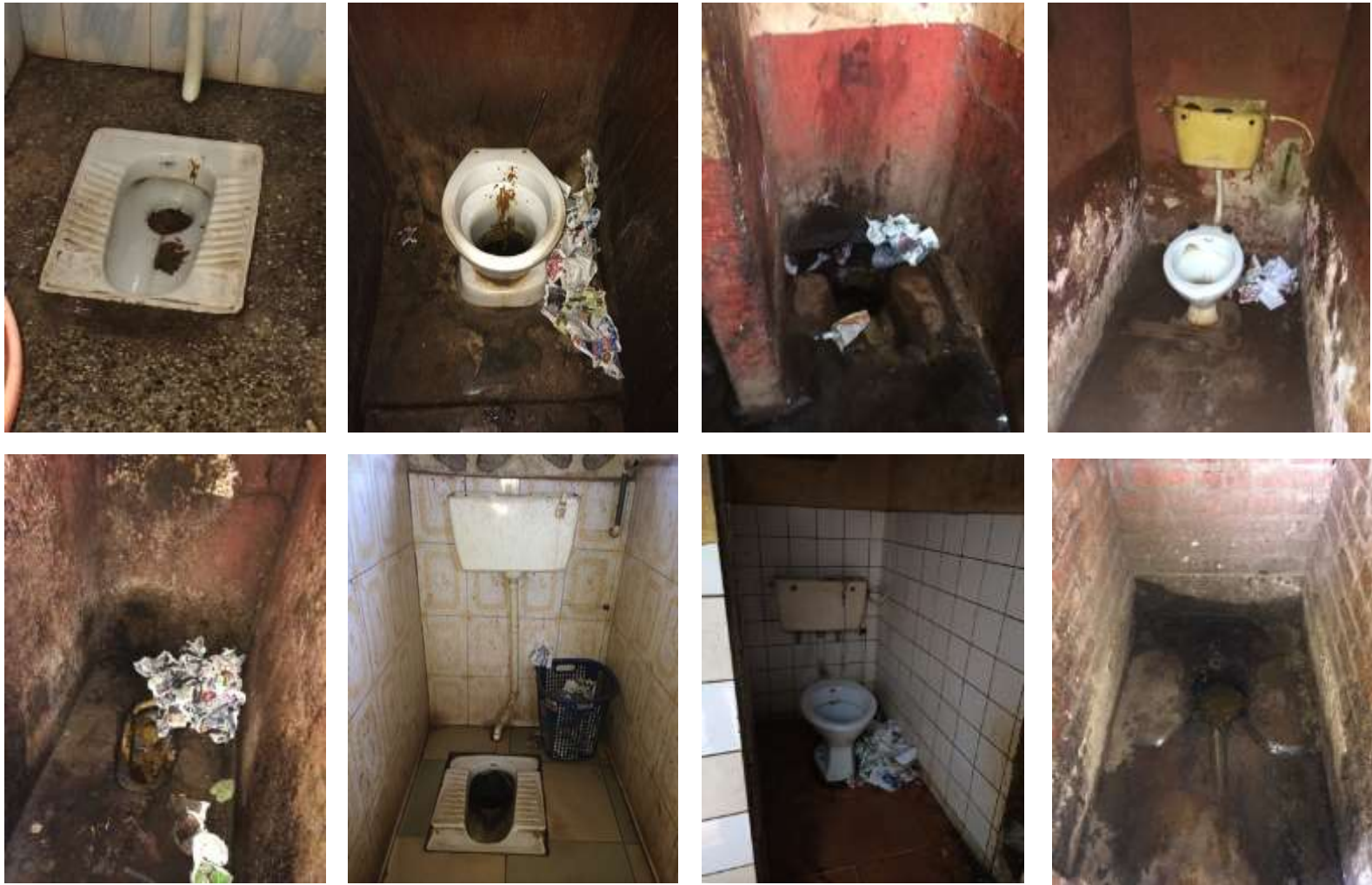
Figure 70: A look in on the condition of public sanitation in CTT's service area in Kumasi (Knutson 2014).
