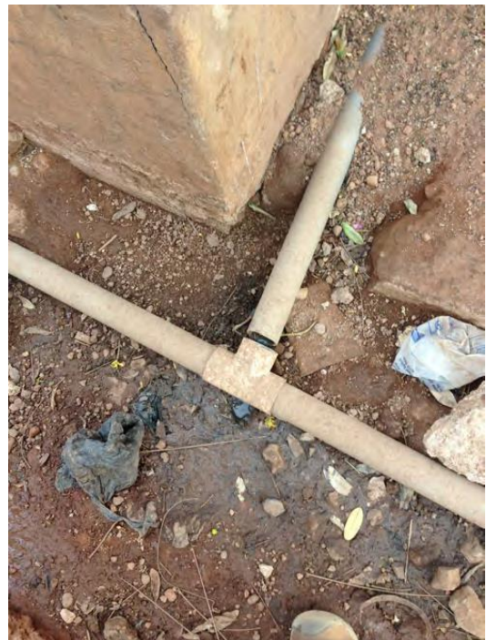
Figure 4-16: Broken distribution pipe (Photo: Deborah Vacs Renwick)
