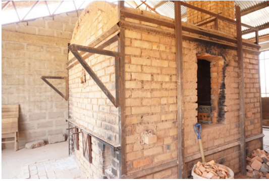
Figure 3-22 The kiln in PHW
